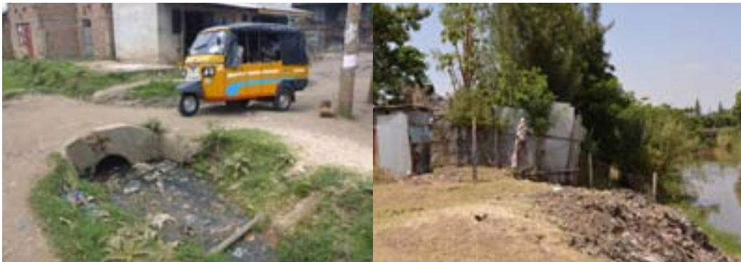
Figure 11 Blocked drainage (l). Pit latrines located along Nyando River (r).
